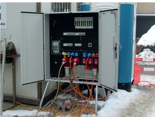
Main distributor on a construction site
